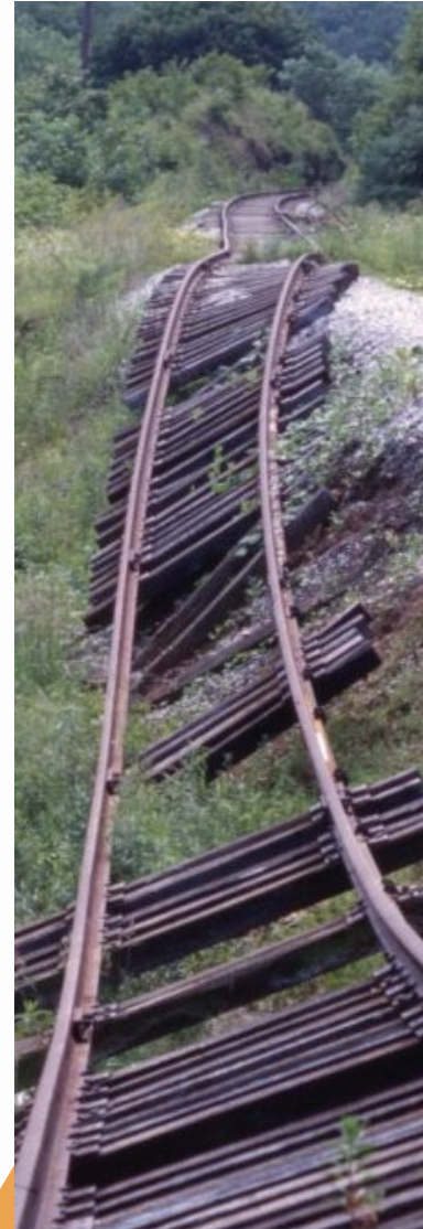
Figure 5 - Damaged Railroad in Carroll County, MD
