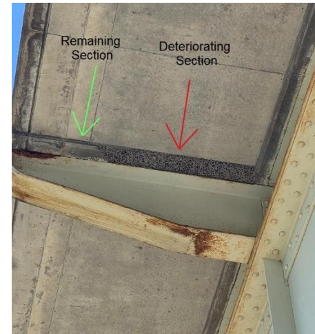
Figure 11 Deteriorating Underside of the US 522 Bridge 210124001 with Falling Concrete Spalls That Pose a Safety Concern for Road Users on Limestone Road
