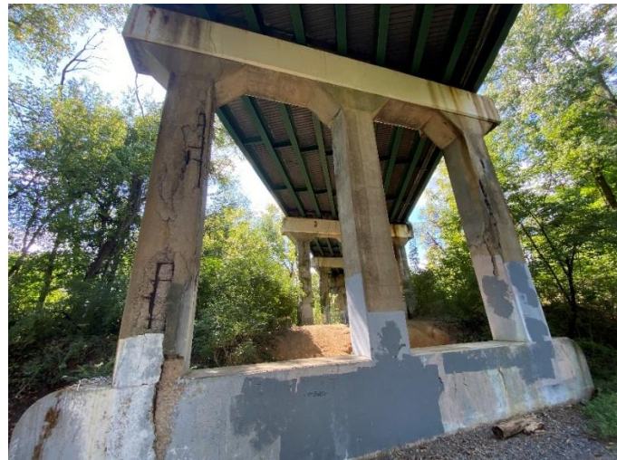
Figure 15 Exposed Substructure of the US 522 Bridge 210043001Is Vulnerable to Floodings Events
