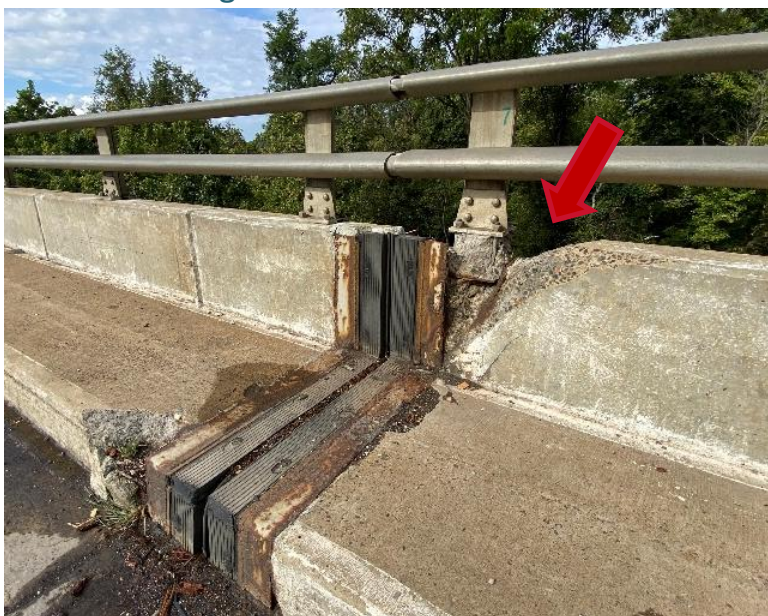
Figure 8 Broken Railing and Blocked Drainage on the US 522 Bridge 210043001
