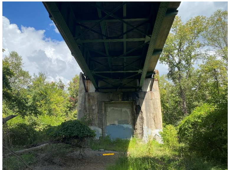
Figure 9 Deteriorated Columns under the Bridge Deck on the US 522 Bridge 210043001
