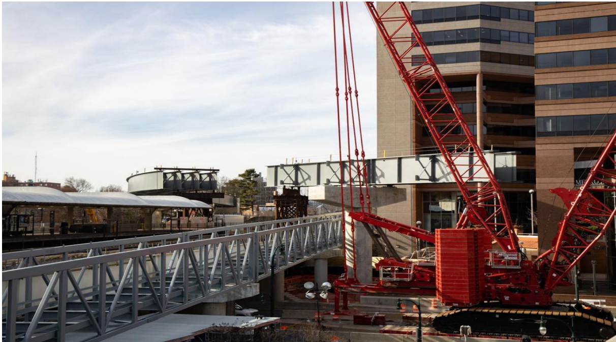
Girder Installation at the Paul S. Sarbanes Transit Center in Silver Spring
